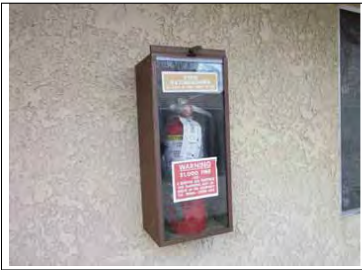
19. Handheld fire extinguisher.
