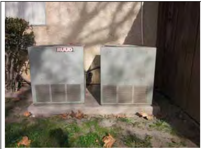
21. Pad-mounted condenser units.
