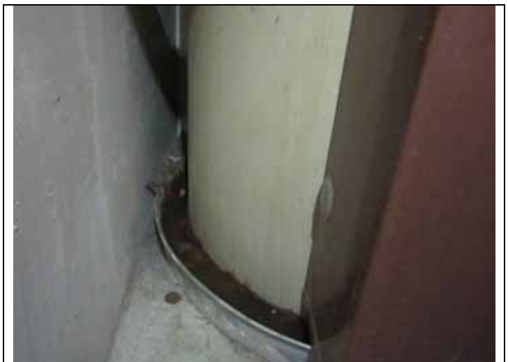
36. Water in the drip pan at Unit 3 water heater indicating leak.
