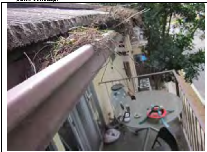
60. Debris accumulated in the gutter along the west side of the building.
