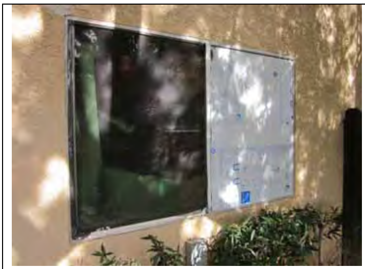
56. Broken window replaced with plastic (Lexan) sheet at southwest corner of the building, Unit 4.
