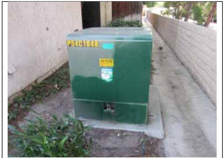
12. Pad-mounted electric transformer.
