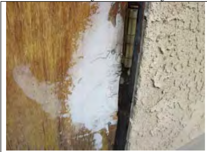
47. Damaged door at Unit 2.
