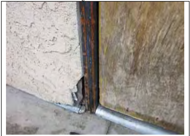
48. Example of typical stucco damage observed near door framing.
