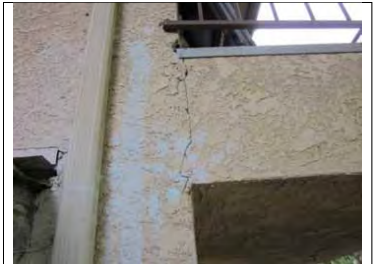
52. Stucco cracking at the northwest corner of the building near Unit 12 balcony.
