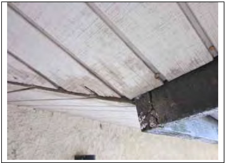
44. Moisture damage at the soffit area at the corner of the building near Unit 9.
