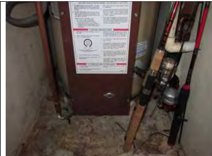
39. Moisture damage at Unit 1 water heater closet.
