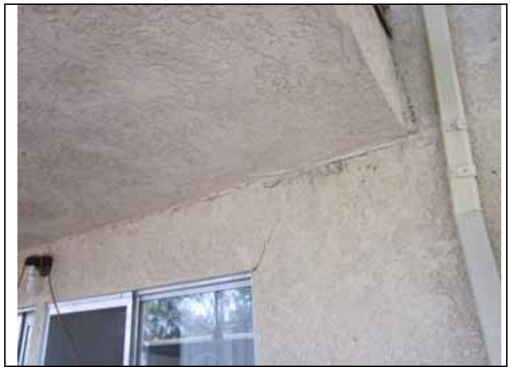
50. Stucco cracking near window framing.
