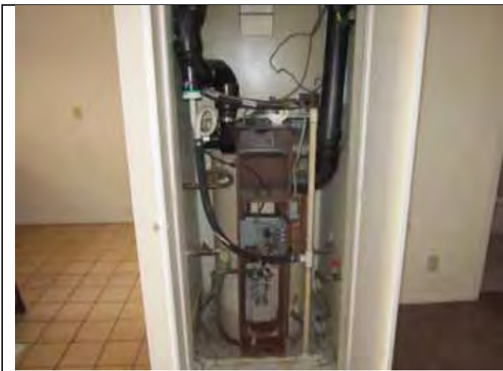
23. Water heater and fan coil unit at interior closet.
