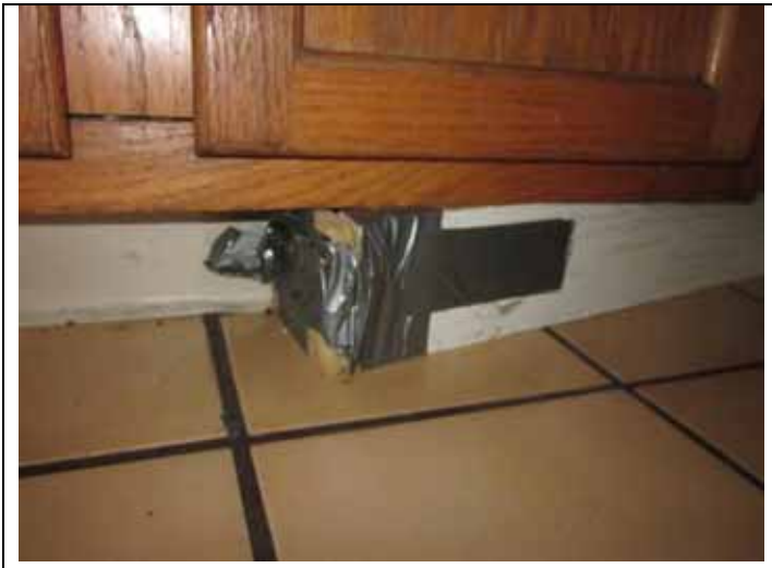
33. Damaged cabinetry at Unit 6 kitchen.
