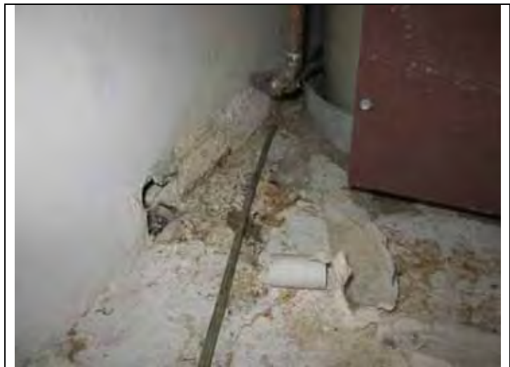
38. Drywall damage at Unit 10 water heater closet.
