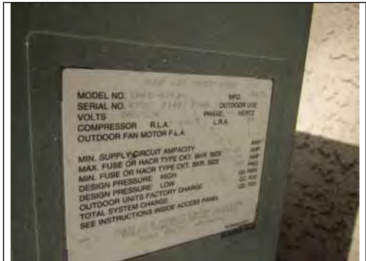
22. Manufacturer label indicating manufacture date of 03/91.
