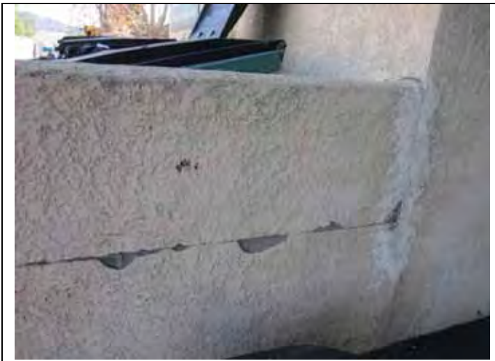
53. Stucco damage at the trash dumpster enclosure wall.
