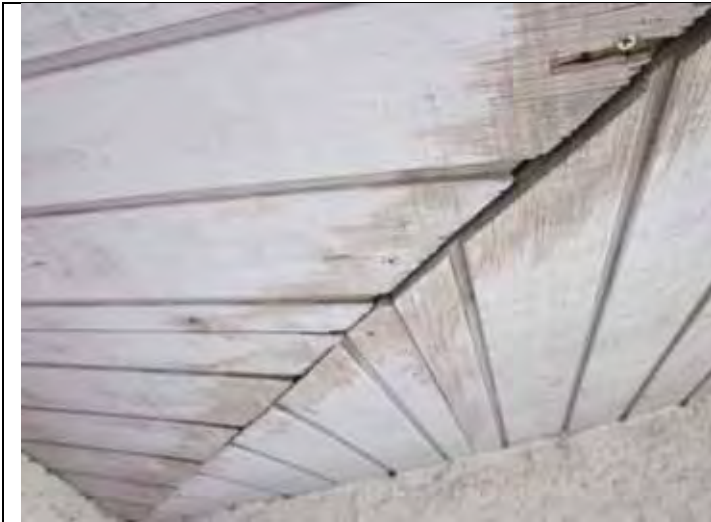
45. Another view of the moisture damage at the soffit area at the corner of the building near Unit 9 indicating roof leak.
