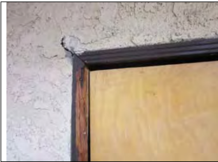
49. Another example of stucco damage near door framing.
