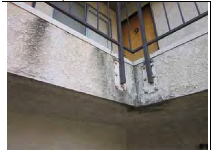
54. Staining typical along the upper level walkway.
