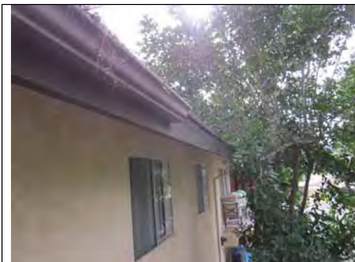
59. Trees in contact with the building along the west side.
