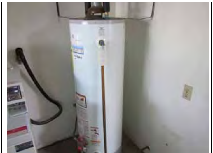
16. Central water heater for the laundry room.
