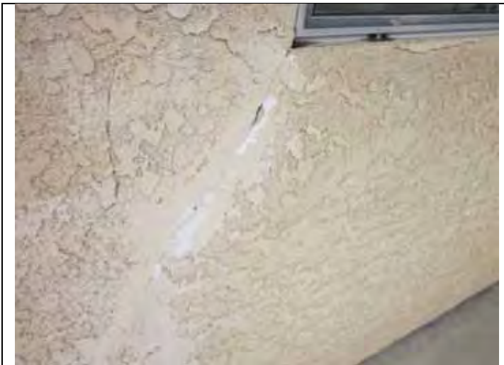
51. Another example of cracked stucco at window framing.
