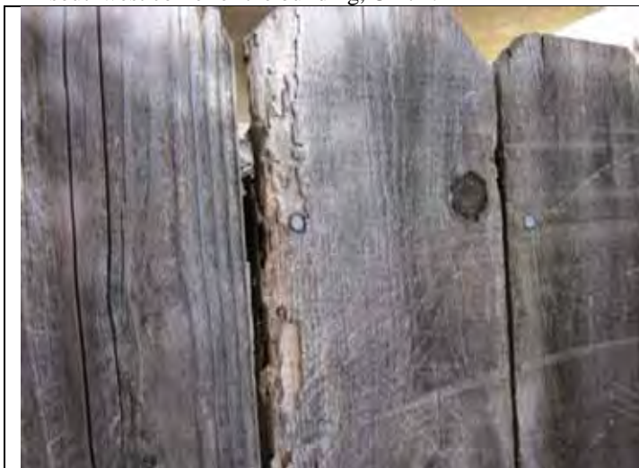
58. Evidence of potential wood-destroying organisms at the patio fencing.
