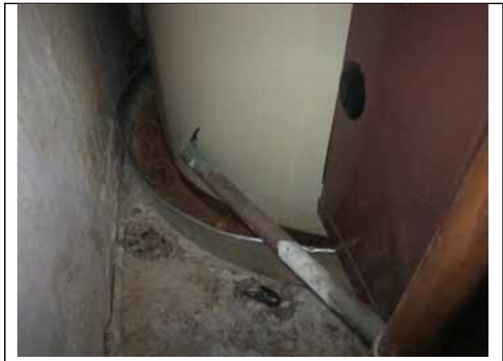
40. Water and corrosion in the drip pan at Unit 1 indicating long term leak.
