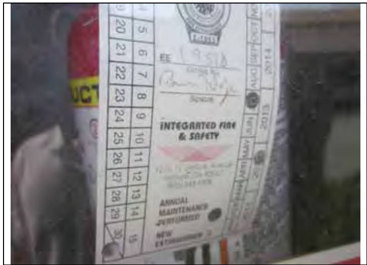
20. Current inspection tag for the fire extinguisher.
