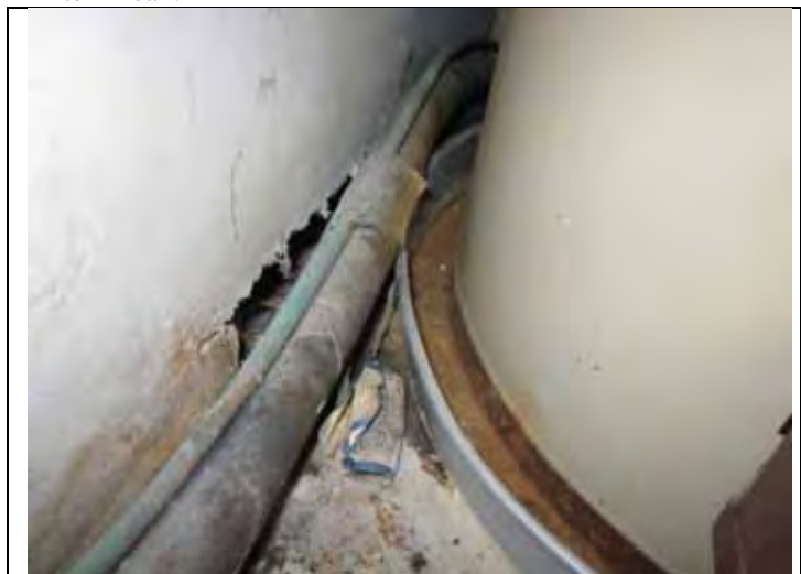
42. Drywall damage at Unit 6 water heater closet.
