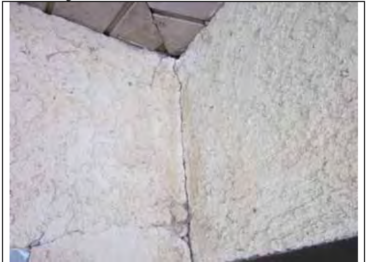
46. Stucco damage and moisture staining near the soffit area at the corner of the building near Unit 9.
