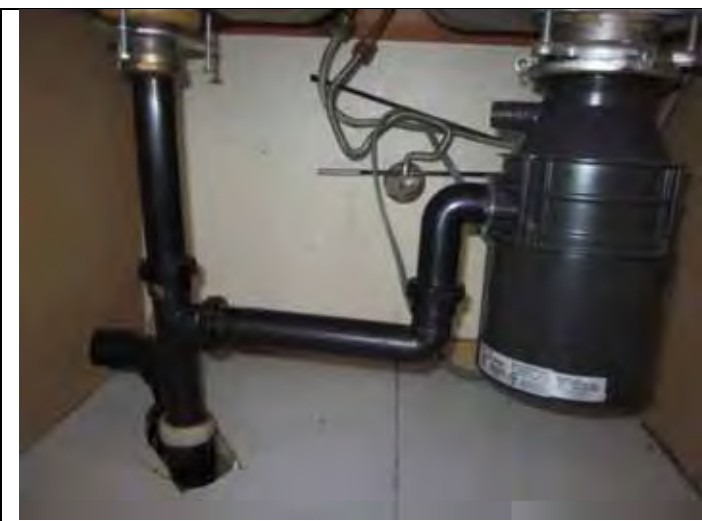
29. Under-sink plumbing with garbage disposal.
