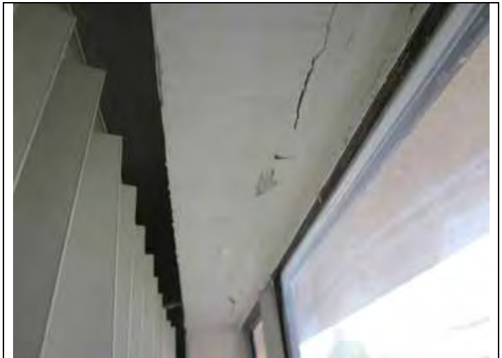
34. Water damage at Unit 3 bedroom upper window framing.
