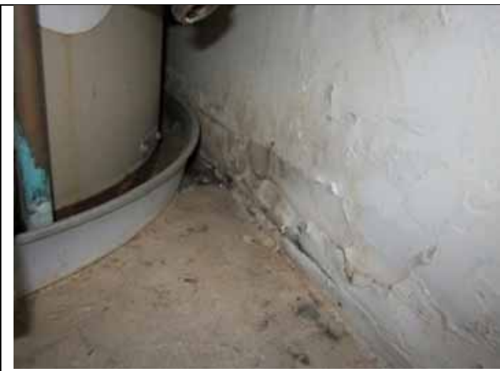
41. Moisture damage at Unit 6 water heater closet.
