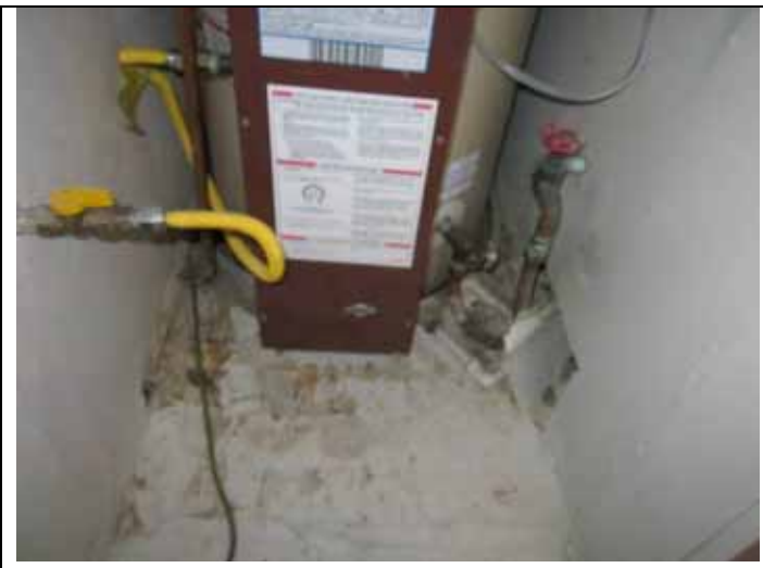
37. Moisture damage at the water heater closet floor at Unit 10.
