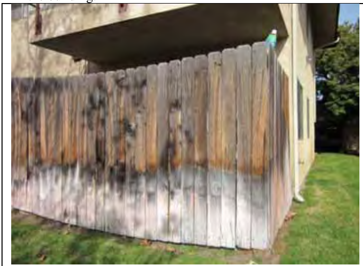
57. Example of wood damage typical at the patio fencing.
