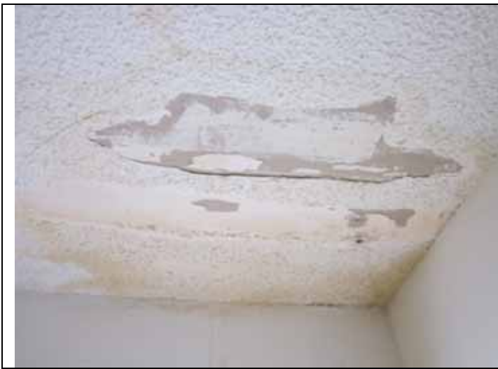
43. Moisture damaged ceiling at Unit 9 entry.
