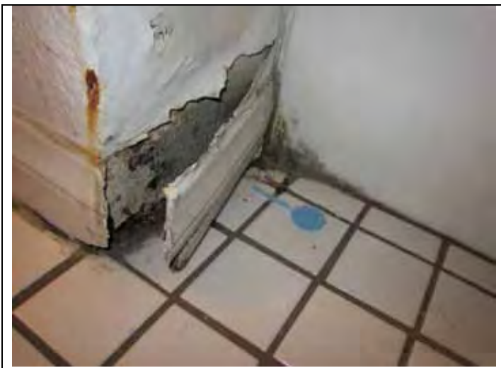
35. Water damage at Unit 3 bathroom near base of the tub.
