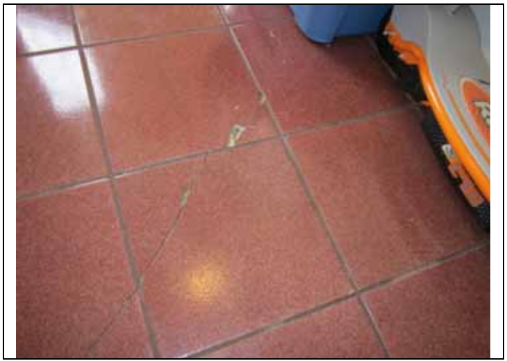
32. Damaged flooring at the entrance to Unit 1.
