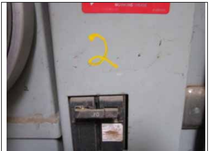
14. 70-amp service to each unit.
