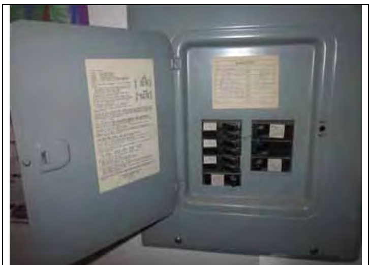
30. Electric subpanel with labels.
